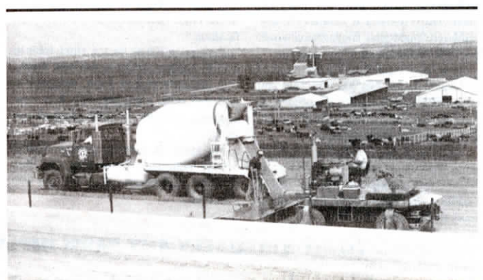
The first day workers used new machine they laid 820 ft. of solid concrete feedbunk.
