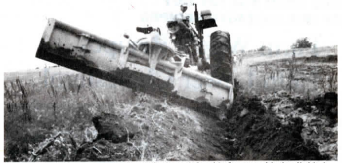
It takes about three passes to dig a 3-ft. deep, 3-ft. wide furrow with the tilt blade.
