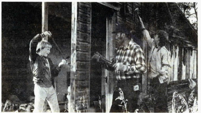
The Roberdeaus pry off each board with tender loving care to avoid marring or splitting.
