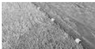
Plastic clips made from short sections of pipe are used to clamp plastic to pipe.
