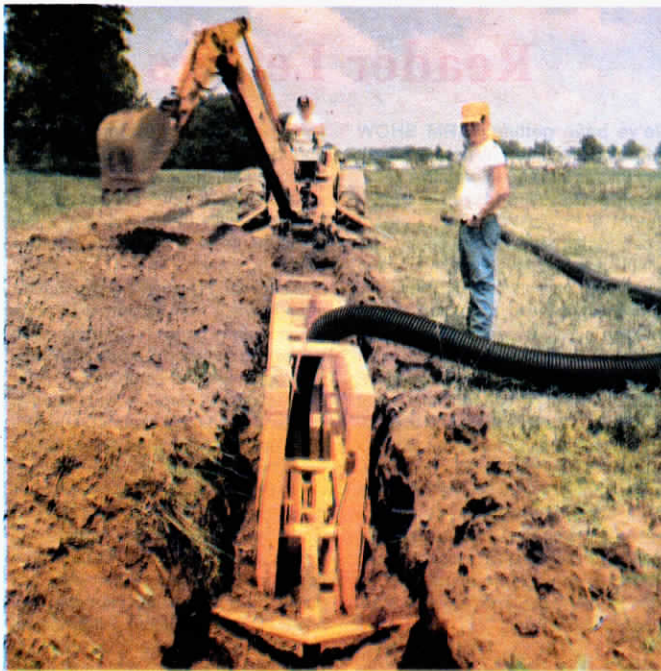
Pull-A-Long unit, set into bottom of a 24 in. wide trench, automatically cuts the exact grade and lays the tubing as it's pulled along.
