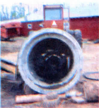
Tire flips inside out as it's pulled into culvert by 4-WD tractor.
