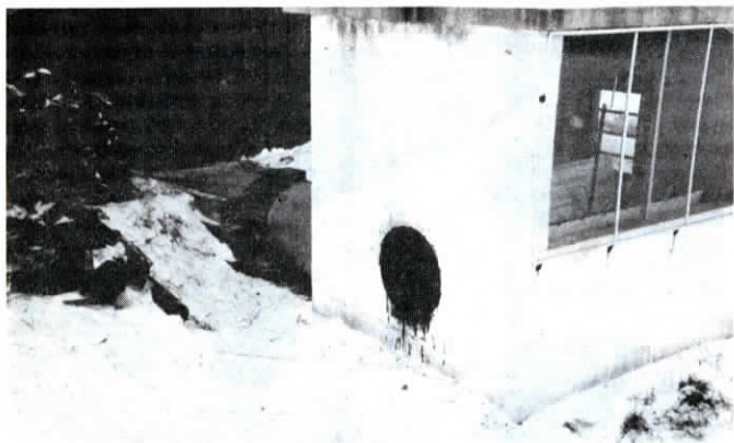
Wood stove is housed inside a 7 by 7-ft. concrete building. An axial vane fan is mounted inside a metal duct that connects furnace room to a metal duct under storage shed.
