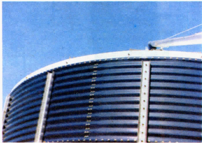
Note the vertical "stiffener" braces, made of U-shaped channel iron, located about 50 in. apart around the outer bin wall.
