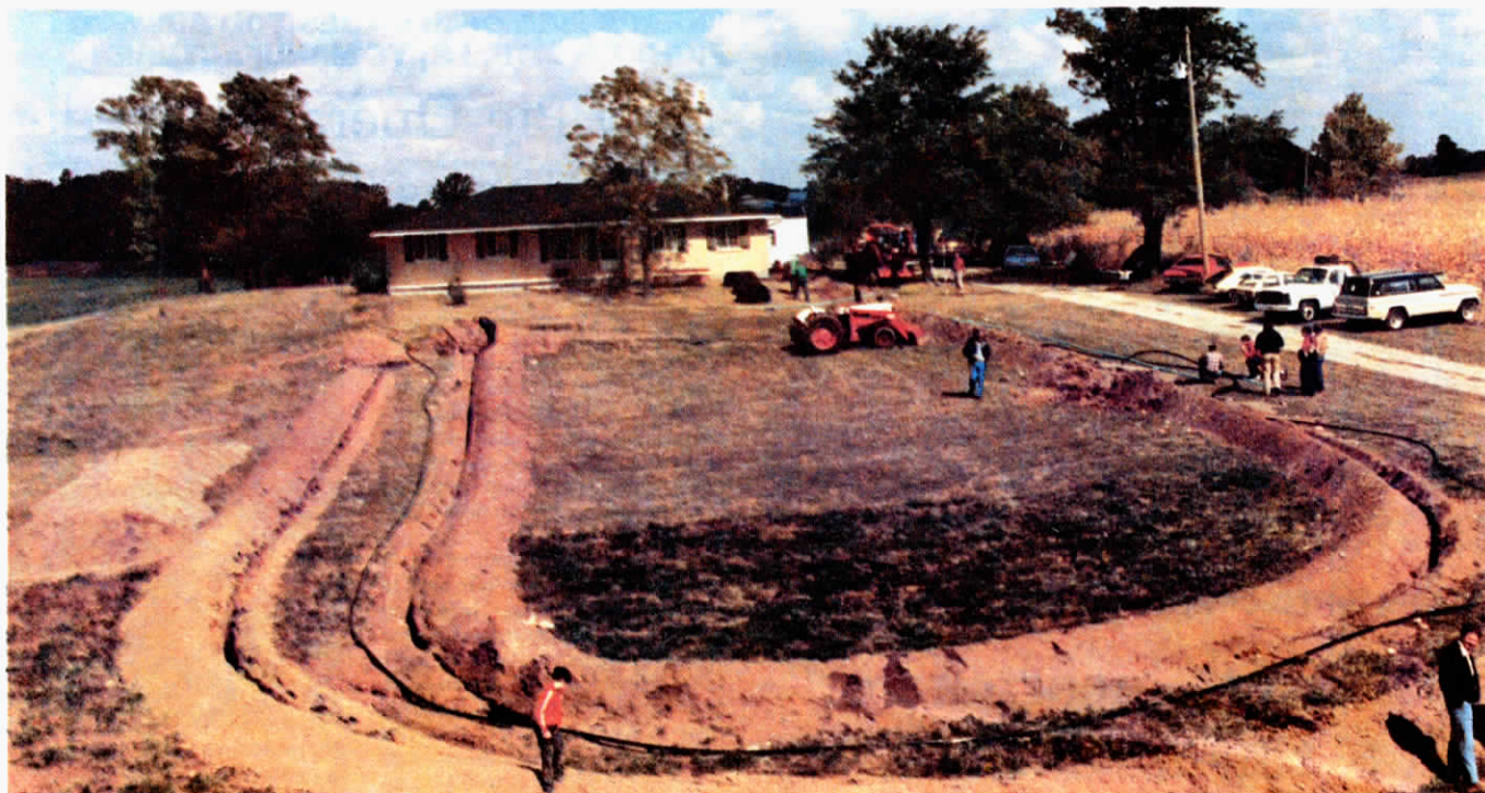
Underground heat, picked up by a water/methanol solution circulating through buried pipes, heats the Clark home in winter. The same system cools the house all summer.
