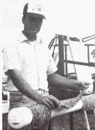
Carpet strips (2 ft. long, 1 ft. wide) are "stuffed" 6 in. into pipe groove, with 6 in. of carpet left on outside of pipe.
