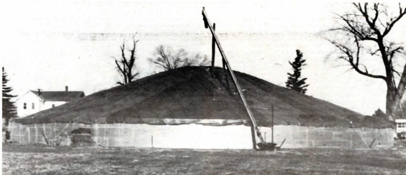
A special "catenary" cable and grommets secure the tarp to a circular metal ring.
