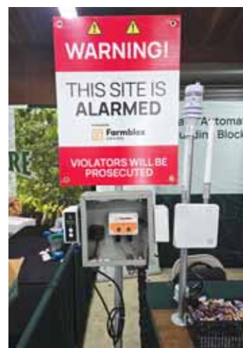
Security system integrates with control panels and supply lines on wellheads, irrigators and other equipment, instantly sounding alarms and notifying owners and law enforcement when tampering occurs.
