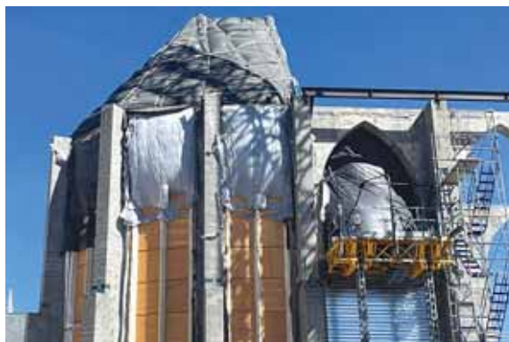
Old parachutes were used to create a weatherproof cover to continue construction.
