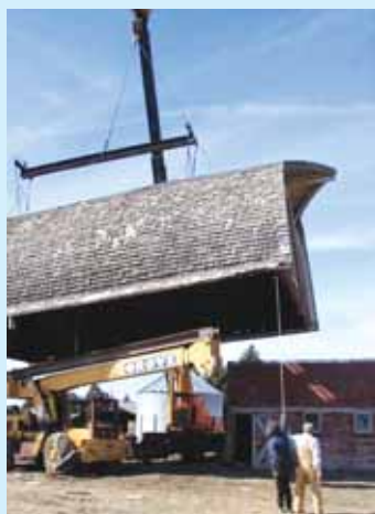
A huge crane lifted the roof from the supporting walls for the move.
