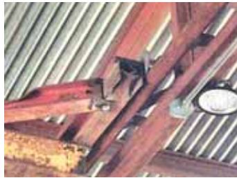
Surber built an overhead bridge crane for his shop that rides on rails made of oilfield pipe.
