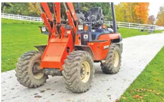
4-ft by 3 1/2-ft. ground protection panels float over uneven and soft ground and lock together to support heavy vehicles.
