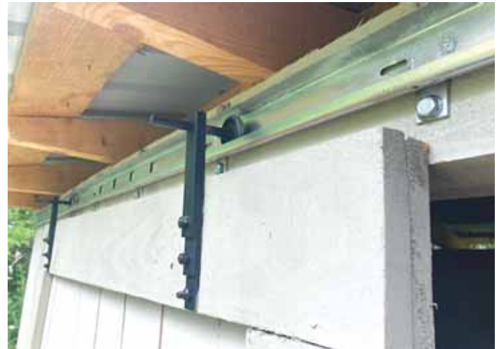
Stoloski used old garage door parts to make a track system for outbuilding doors.
