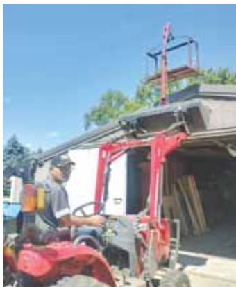
Boyles built a boom lift for his loader to lift shingles to a roof and now uses it for many other jobs that "save his back".
