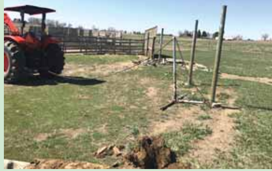
Chain is hooked to the end of the pipe on the ground and wrapped around the post and up through the eye on the vertical pipe to the tractor hitch.
