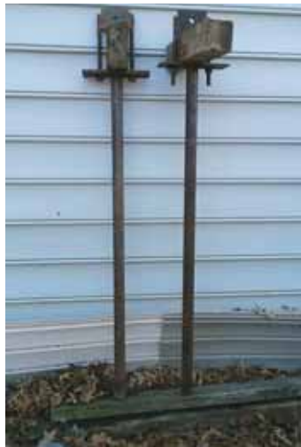
Adjustable 12-in. long bolts are used to tighten two 1/2-in. thick steel plates together against 4 by 4 post to straighten it out.
