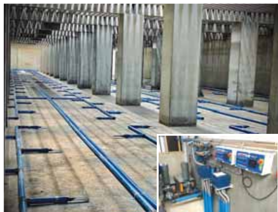
Aeration system pumps oxygen through pipes to keep slurry continually agitated and ready for pumping. It also eliminates the buildup of dangerous gasses.
