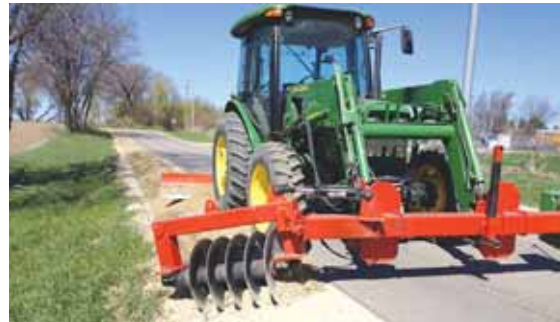
Loader-mounted “reclaimer” uses a series of big coulters to reclaim lost shoulder gravel from ditches.
