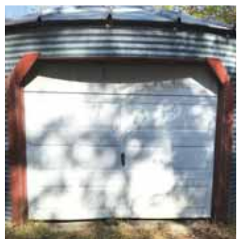
Garage door sets inside a 2 by 4 wood frame, with the overhead track supported by another wood frame.
