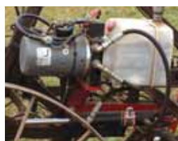
Hydraulic pump and reservoir.
