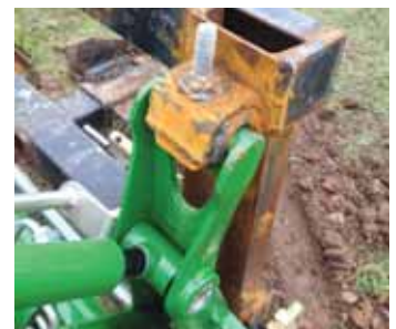
Wideman welded quick-tach mounting brackets to frame’s upper corners, then closed up a hole in each bracket’s reinforcement plate by welding a bolt into it.
