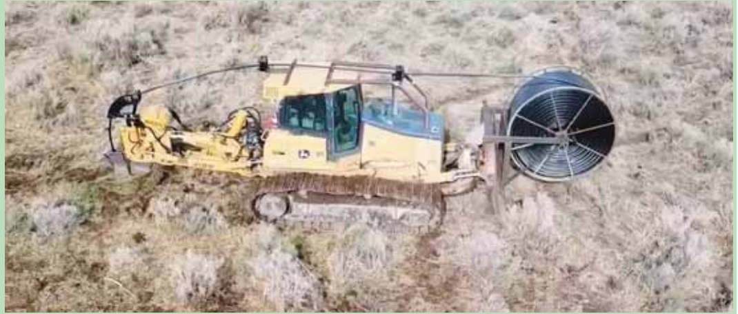
Joe Heaton installs underground HDPE pipe to help ranchers develop springs and ponds into permanent watering systems. He uses a dozer to pull a vibrating plow and attaches a reel carrier to the blade.
