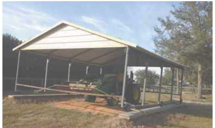
Weller ran the front chain through an 8-ft. long piece of square tubing that’s secured to the loader bucket with ratchet straps.
