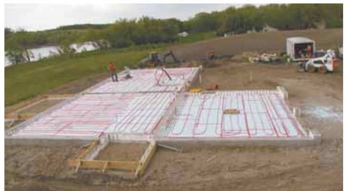
When needed, winter heat is provided by a ground source heat pump and in-floor heat, which extends into the garage.
