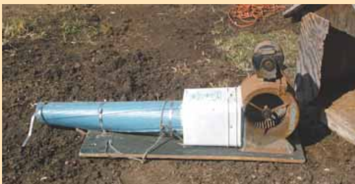
A squirrel-cage fan blows air through a makeshift funnel into the pvc pipe aerators. A timer turns fan on and off periodically.
