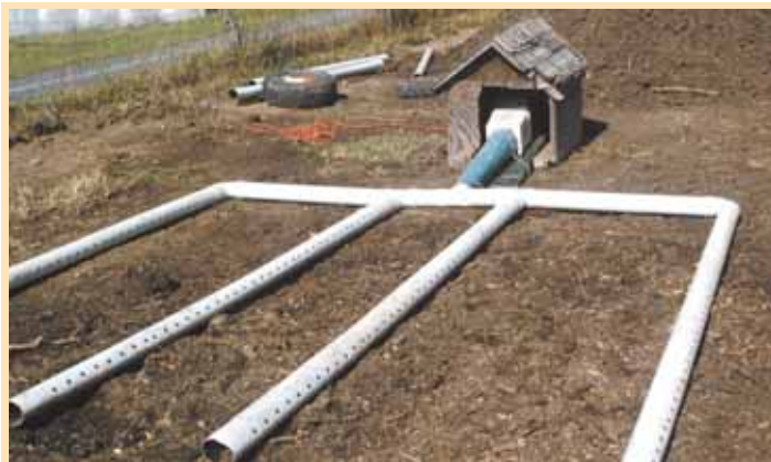
“Static pile” method of composting eliminates the need for stirring. Four 30-ft. lengths of 4-in. dia. pvc pipe are connected to a cross pipe “manifold” attached to a squirrel cage furnace fan.
