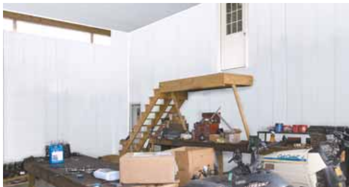
EconoPanels were recently installed on the walls and ceiling of this new 2-story repair shop.
