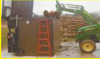
Outside Boiler Burns 9-Ft. Logs (Page 17)
