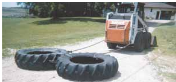
George Klose levels his driveway with 2 big tractor tires, running cables through the tires and over the top.
