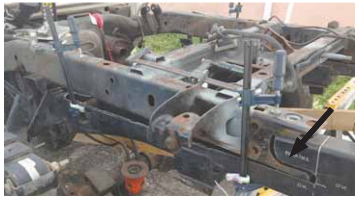
When Kazmierczak bought a Dodge Ram 1500 pickup at an auction, he planned to lengthen the frame in order to fit a utility bed he already owned. Arrow shows where frames were cut to fit together.
