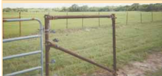
To reinforce his gate posts, Russell Hackman made brackets that allow him to attach diagonal or straight-across rails to vertical posts.
