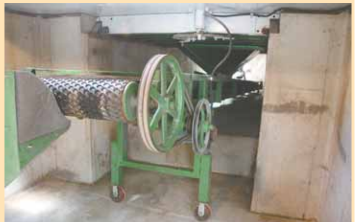
Kelly and sons reduced costs by designing and building many components including this movable pit conveyor that’s mounted on wheels.
