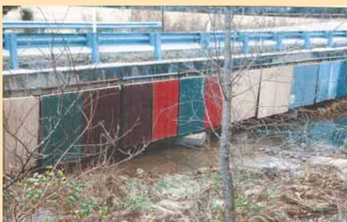
A series of tin panels pivot backward when the water rises, and then fall back in place as the water recedes. Brush and debris wash on through.
