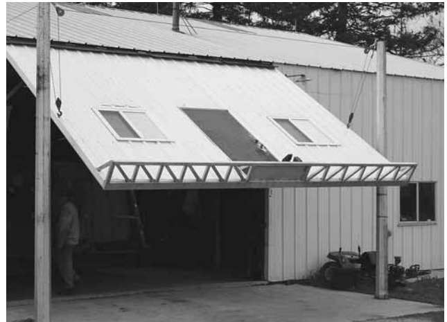
Virgil Pook replaced the worn out door on his shop with a flat panel that has walk-through door and windows.
