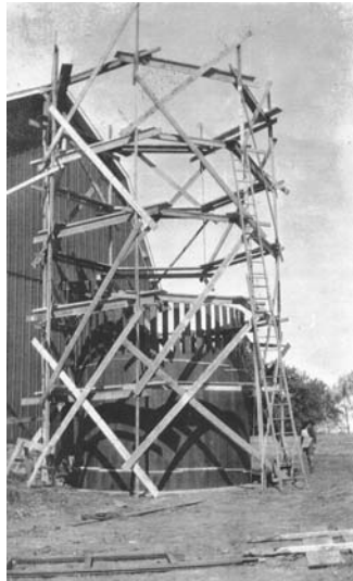
Photo above was taken in 1915 and shows the silo being constructed inside a circular wooden scaffold.
