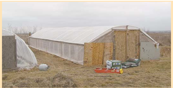
He closed off the tunnel's north end with plywood and a 4-ft. door that can expand to an 8-ft. door. Tunnel's other end is closed in.
