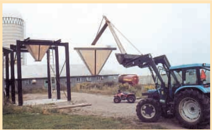
Carrier's 32-ft. tall structure houses four bins made from 1/2-in. plywood.
