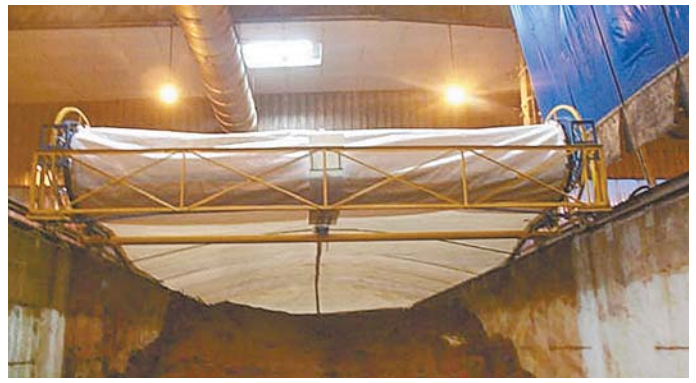
Airtight cover allows all odors and gasses to be pulled off for processing. Cover can be retracted temporarily whenever compost needs to be turned.
