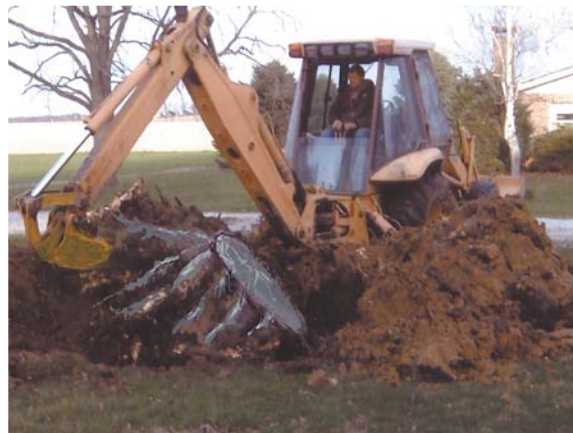
Using a backhoe to dig out tree stump allows ground to be more easily leveled off and reseeded.
