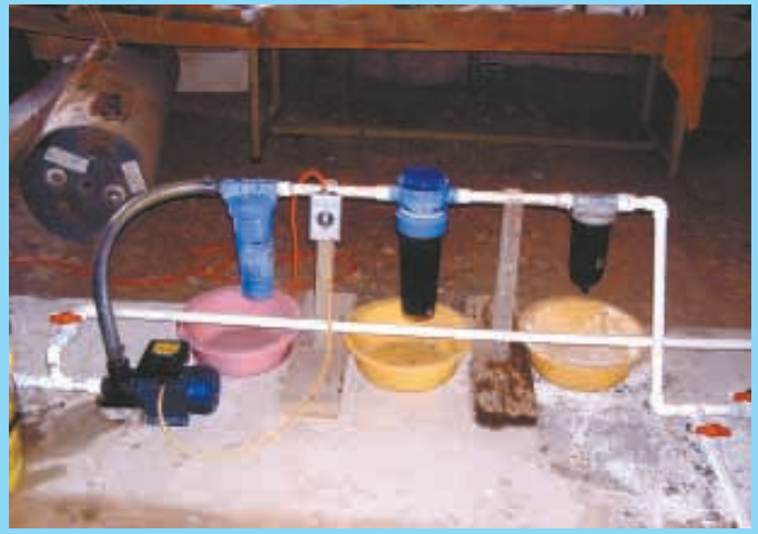
System consists of a 300-gal. bulk tank and two 55-gal. barrels spaced about 15 ft. apart. A 12-volt pump with a filter and valve system are positioned between them.
