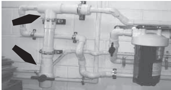
Ponder installed a larger section of pipe in water line (see arrows) to catch grit before it reaches filter. Spigot at bottom is opened to eject grit.
