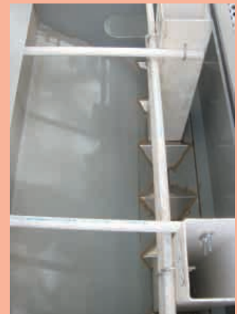
U-bolts secure two lengths of 1/2-in. pvc pipe to each pair of box inserts.
