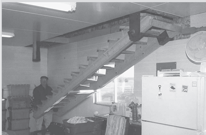
"It lets me carry big, wide objects up into my loft," says Ray Rowden, who made this 30-in. wide staircase for his shop. It's raised by an electric winch (not yet installed when photo was taken).
