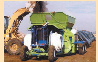
A machine similar to a silage bagger pushes waste material into plastic bags called "pods".
