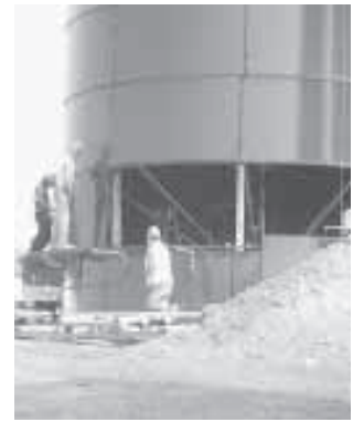
Photo shows Penn Jersey workers putting up a used 25 by 80-ft. Harvestore.
