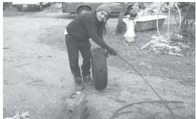
When done cleaning sewer pipe, Hicswa coils line inside tire for storage.
