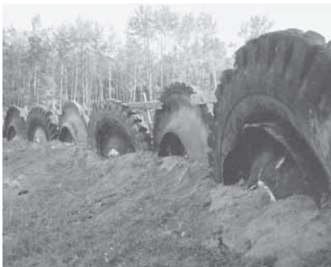
"Tire fence" was built out of 9-ft. high earth-moving tires set in a 12-in. trench. Soil was backfilled into trench about 18 in. above ground level.
