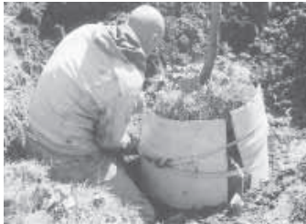
After digging trench around tree, Marley straps plastic barrel halves to it.
