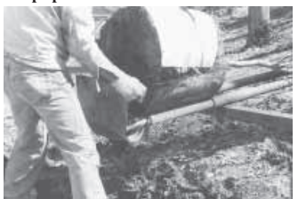
Wrapped tree is strapped to cradle and then a steel plate is inserted into bottom of tree mover to hold tree in place when it's set into new hole.
